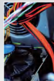
Transformer line inspection
